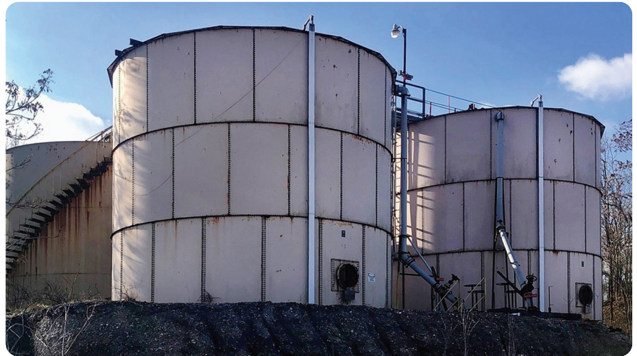
Out-of-service equipment like these empty storage tanks will be removed from the facility's hazardous waste permit.
